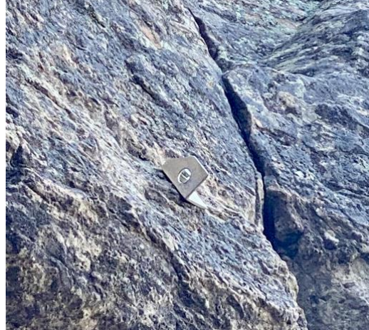
Figure 4: A dangerous old homemade aluminum L-stock hanger used on the first ascent of a climb in Southwest Colorado. These types of bolts are in need of a safer replacement with new age \frac{1}{2} inch steel bolts.
